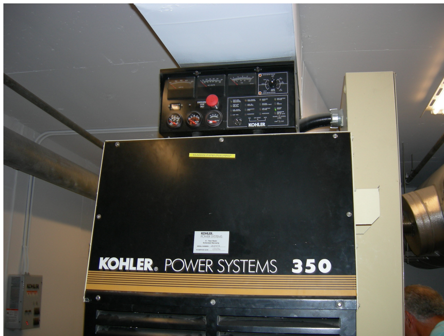
Figure 2.3.1 Savoy Motor-Generator Set-Front View
